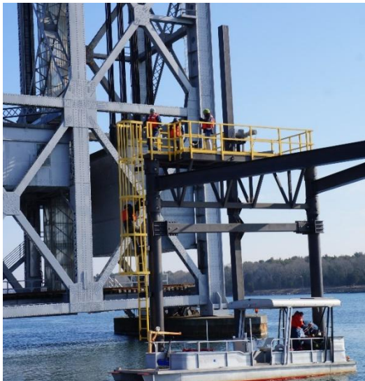
Caption: URI and MRECo crew installing water level sensor atop the BTTS Platform.
